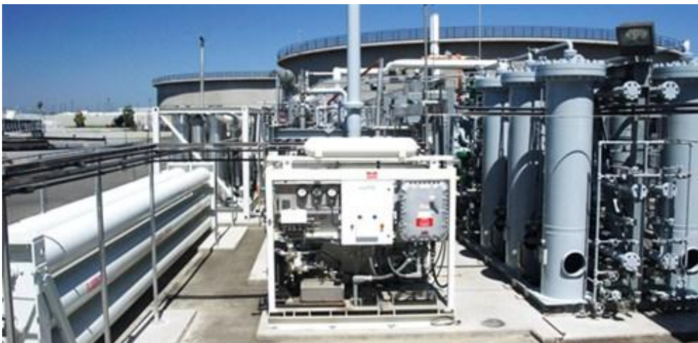
Air Products' Orange County wastewater treatment plant (Source: Air Products)
